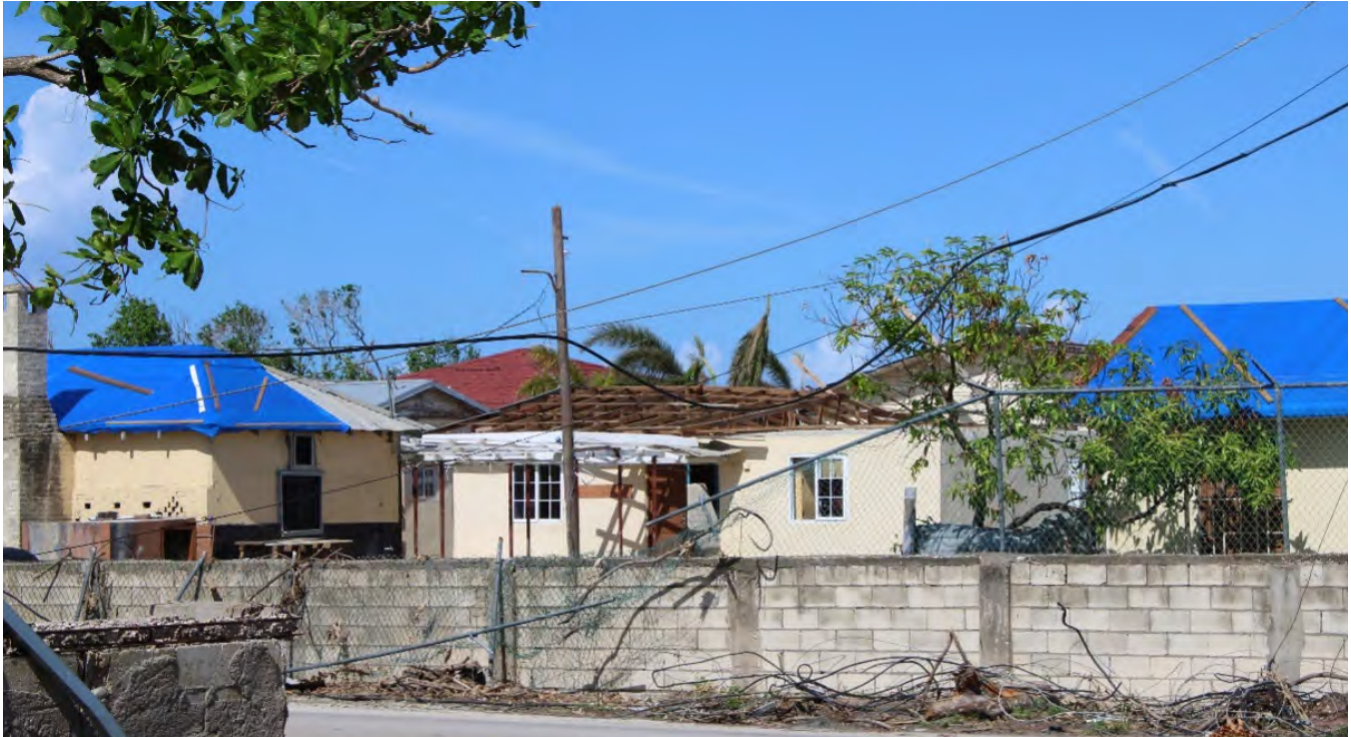
The Trelawny Infirmary which was damaged by Hurricane Melissa.
